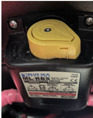
Image 12: Battery Switch Locked Off
