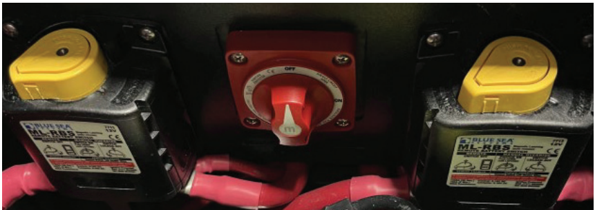
Image 4: Battery Box Battery Switches in Remote OFF
