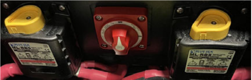
Image 3: Battery Box Battery Switches in Remote ON
